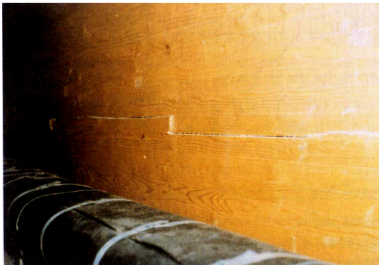
Fig. 9. Longitudinal through crack in glulam roof girder due to shrinkage effects. Hot water piping in the vicinity of the girder contributed to fast drying. Source: Ref. [7].
