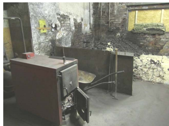
A “dirty” boiler and accompanying coal supply.
