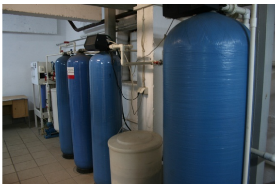
Water purifiers in a gas-power boiler plant operated by OPEC.
