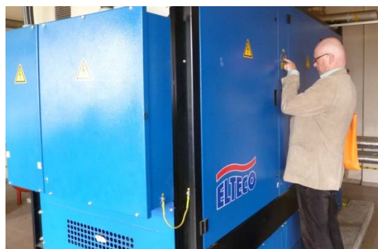
Electricity generation by a diesel engine fuelled by biogas.
