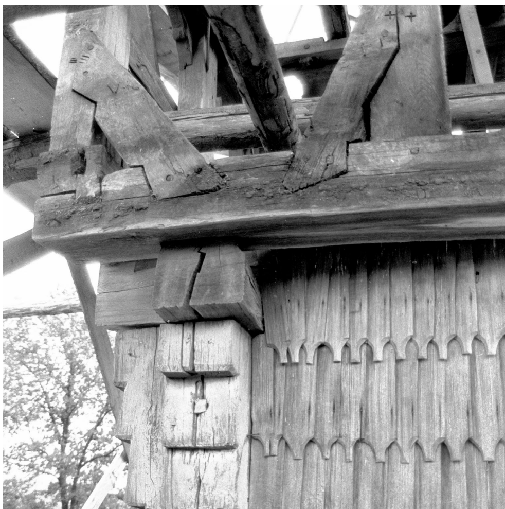
133 Desești . During the repairs from 1996, the hidden parts of the tower were exposed revealing numerous assembly marks of great variety. Here there can be observed the graphic signs “+” and “III” on both the gallery posts and their respective downward angle ties. Unfortunately, some of them were lost with the replacement of some original pieces and some due to the “cleaning” of the surface with an axe without any thought for their historical value. Photo: June 1996.
