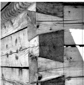
40 Dragomirești. The settlement gaps were plainly visible during the construction of a new wooden church in Dragomirești by master carpenter Găvrilă Hotico Herenta from Ieud. Photo: July 1997.
