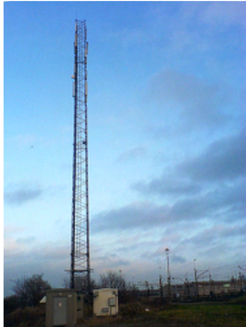
Mast in Malmö shared by Svenska UMTS (Telia Sonera/tele2) – using it for both GSM and UMTS, Vodafone (Telenor), and Tele2 – using it for GSM.
