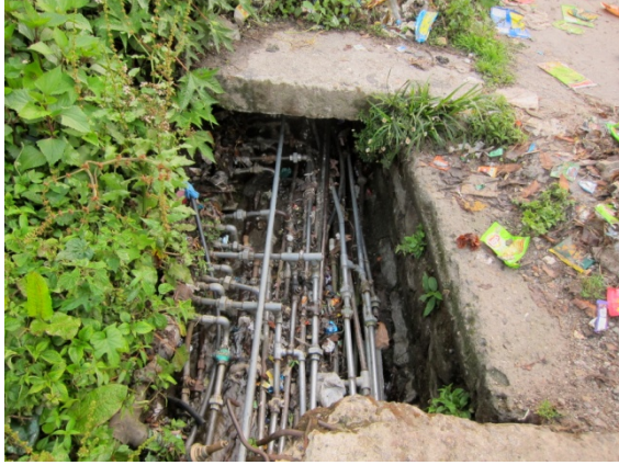
Current pipe and storm water drain infrastructure
