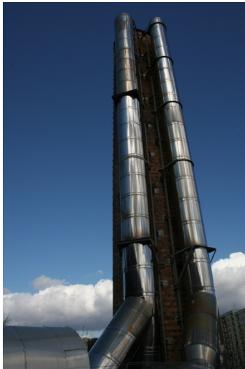
Present and past meet – chimney for one of the gas-power boiler plant operated by OPEC mounted on the old.
