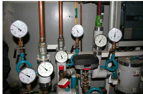
Gauges on a heat exchanger connect to a small gas boiler operated by OPEC.
