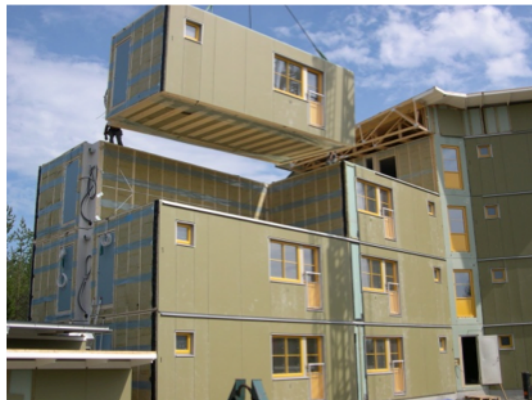
Figure 1 Swedish industrialized production of houses Examples of industrialized house production in Sweden, previously published in paper 1.
