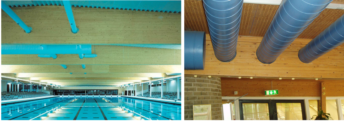
Figure 1.2: Examples of structures with glulam beams with holes. Indoor swimming pool, Västerås, Sweden (with permission for Martinssons Trä AB) and Restaurant Ideon, Lund, Sweden.
