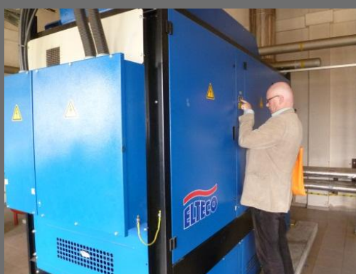
DIESEL ENGINE FOR ELECTRICITY PRODUCTION
