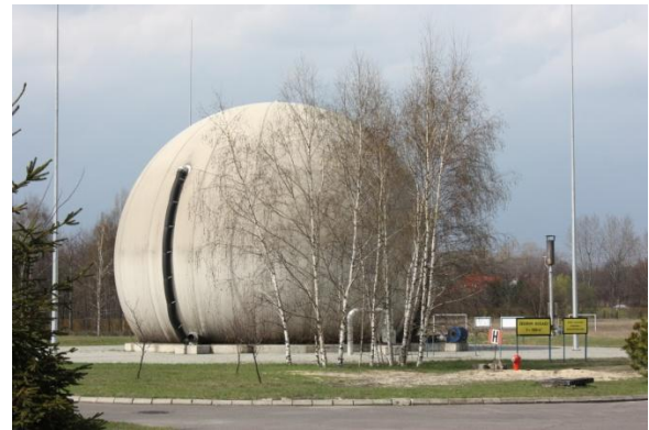
STORAGE FACILITY OF BIOGAS
