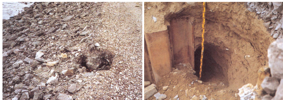
Figure 4. Two examples of effects from internal erosion in Swedish embankment dams. Left: Sinkhole, approximately 0.4 m in diameter, appearing on the upstream side of the crest. Right: Piping, approximately 1 m in diameter, through the dam core adjacent to a sheet pile. Foto: Gösta Johansson, AIB (WSP).
