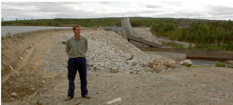
Figure 24. Hällby dam during the reinstallations of electrodes in 2005. The top of the right dam crest is excavated and new electrodes are being placed out, every second being a non-polarisable (white bags). The downstream slope has been reinforced with additional rockfill. In the background are the spillways, the intake to the power station (high building) and the left embankment dam. Author in front.
