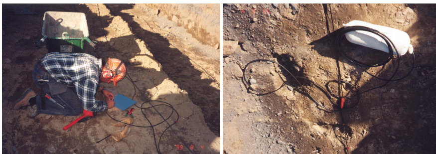
Figure 16. Installation of electrodes at Sädva. Both steel plate electrodes (left) and non-polarisable copper-copper sulphate electrodes pre-packaged in cloth bags with bentonite (right) have been installed.
