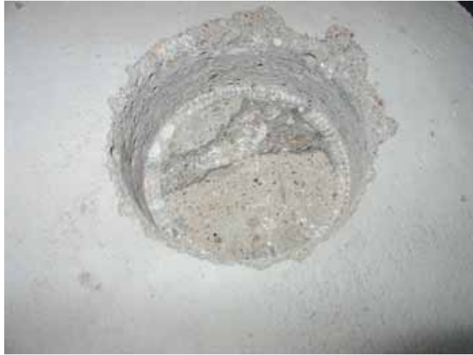
Figure 19. The remaining hole from \text{\O} 90 mm core drill, after extracting samples to moisture distribution determination before flooring. Drilling was performed from the top in a homogenous slab from Batch 1. Note the clear breaking zone separating the mortar screed from the concrete material.
