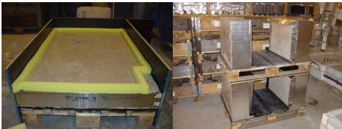
Figure 18. Left picture shows one floor construction in batch 1 prepared for screed application, one corner was spared for sample extraction. Right picture shows four floor constructions from batch 2 vertically tilted in climate conditioned room not yet covered with screed.
