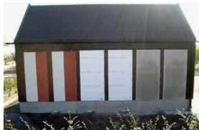
Figure 5.26 The north-facing side of the test house in October 2005. The two façade elements without final rendering are completely wet
