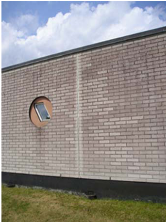
Figure 5.3 Red discolorations on a façade from a building complex in Lund
