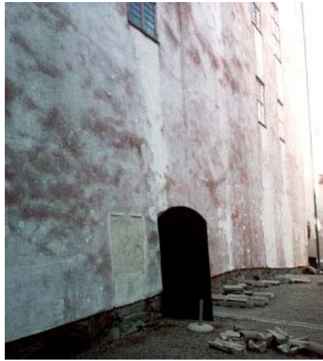
Figure 5.6 Façade of castle in Läckö almost completely covered by Haematococcus pluvialis
