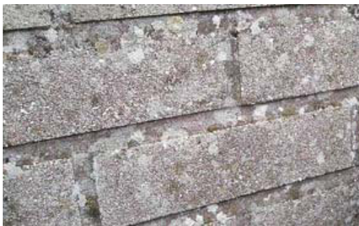
Figure 5.5 Calcium silicate brick wall with growth of several different organisms, mostly lichens
