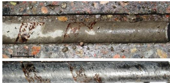
Figure 40. Picture showing corrosion locations at the steel/concrete interface after removing bar 3-A12% (Fig. 37).
