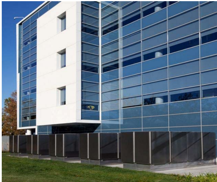
Figur 16. Bloom Energy-stackar installerade hos eBay, © Bloom Energy.
