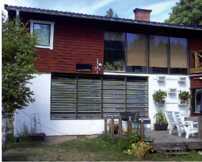
Figure 2.7 The Solgårdens solar window with the reflectors in a closed, vertical, position.
