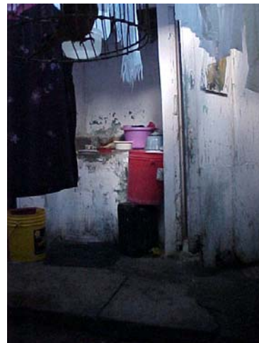
Humidity problems due to leaking roof structures.
