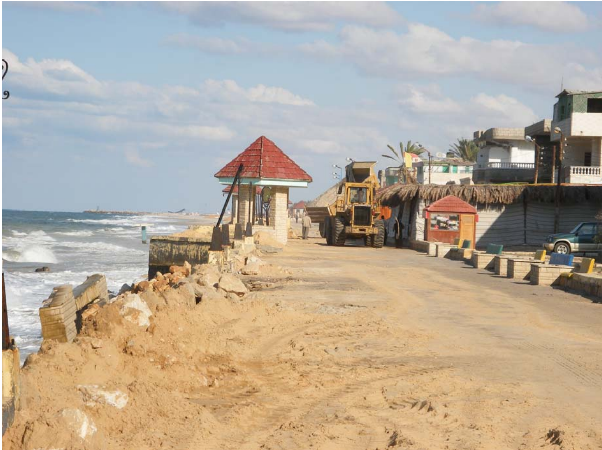
Figure 1.3 Undermining of the revetment 4 km east of El Arish Harbor.
