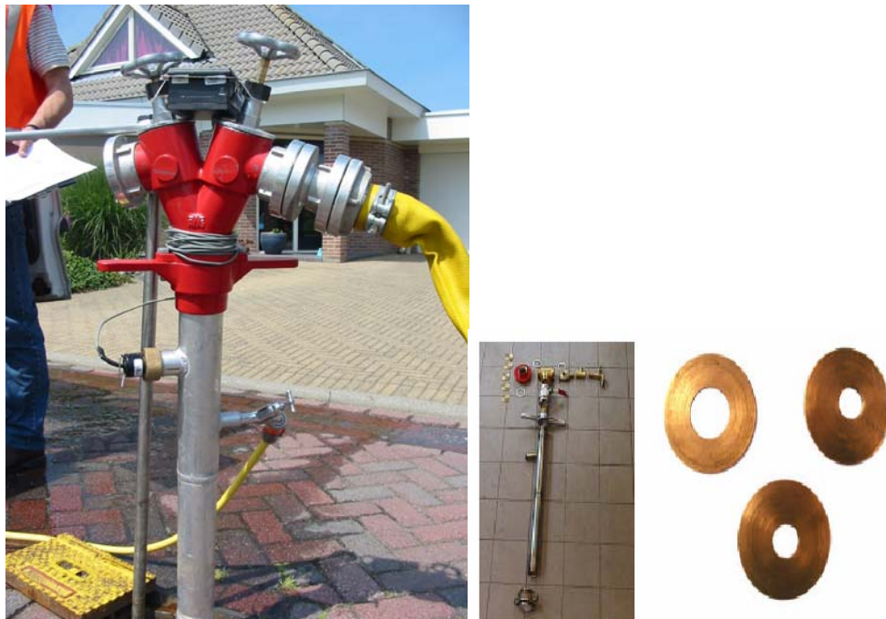
Figure 10 - Example of standpipe setup and ceramic plates used in the Netherlands (left: Kjellberg, 2006; right: Vreeburg et al. 2004b)
