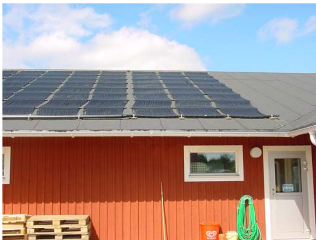
Figure 5-2: Solar heating on the roof of the main building at Ekerums Camping.
