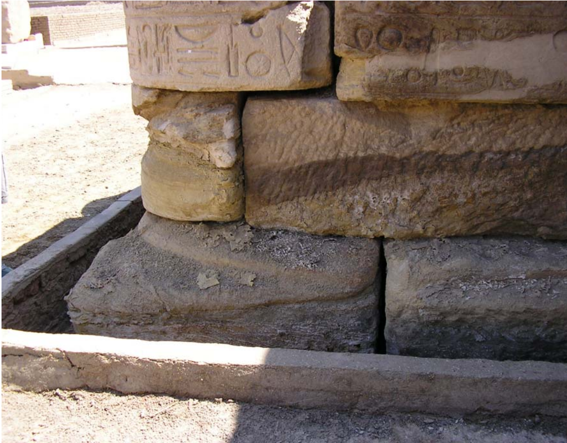
Figure 6: Adverse impacts of water-soluble salts on monuments' foundations and separation of paint and layers of rocks (field trip, Seti Temple, Luxor, August, 2005)
