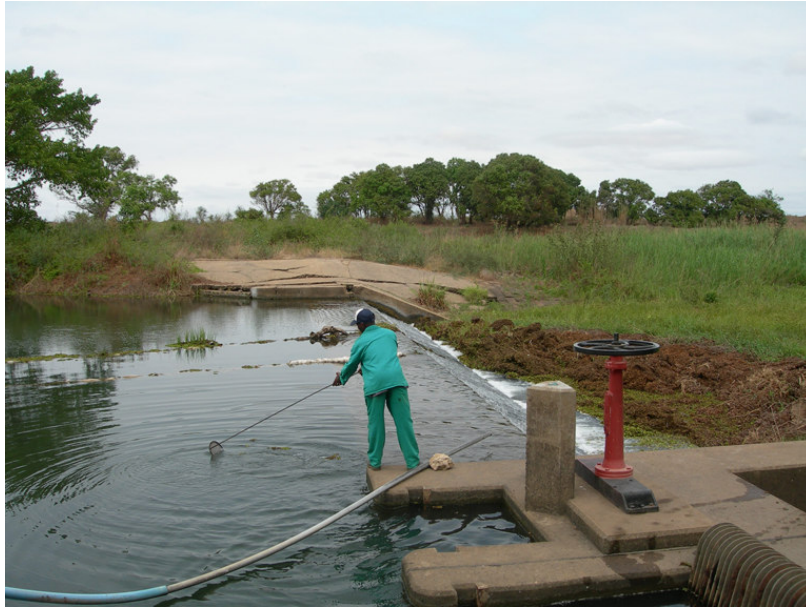
Figure 30 Personnel at the water treatment plant in Boane clear the intake for Salvinia Molesta . On the downstream (right) side of the weir, the River is overgrown with the weed.
