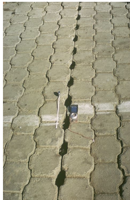
Figure 2.10 A ground rupture in the pavement in the 1972 earthquake.
