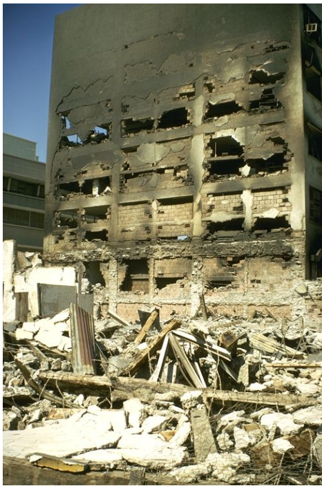
Figure 7.2 This high-rise building has been raged by fire in the 1972 earthquake.
