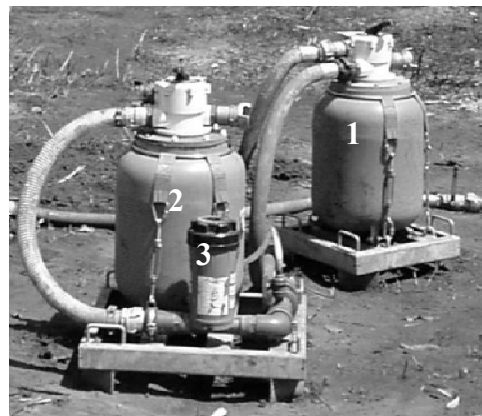
Figure 4.3 Sand 1 and activated carbon 2 filter units and chlorination chamber 3
