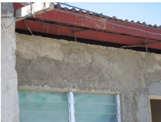
Fig. 10 Ventilation seen from outside, Cabuyao, 2007-04-25
