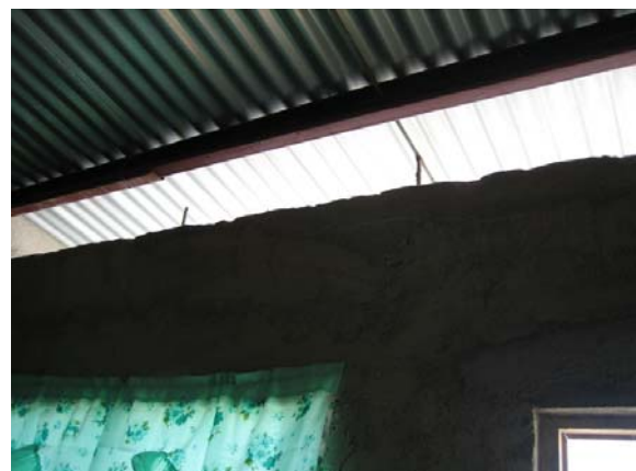
Fig. 11 Ventilation seen from inside, Cabuyao, 2007-04-25
