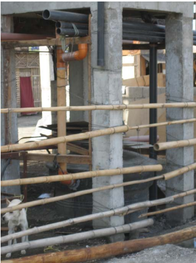
Fig. 31 The septic tank, Sanagmana, 2007-04-28
