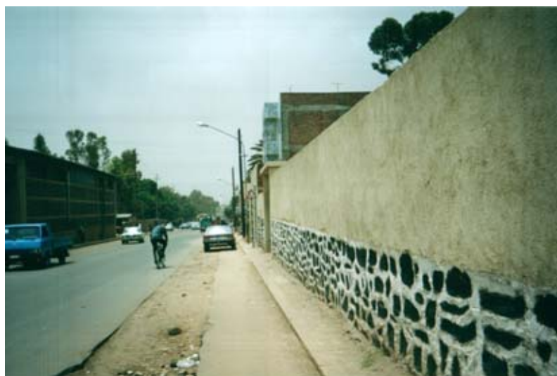
Figure 3.8 Path of gravel after work done on the sewer and drainage system
