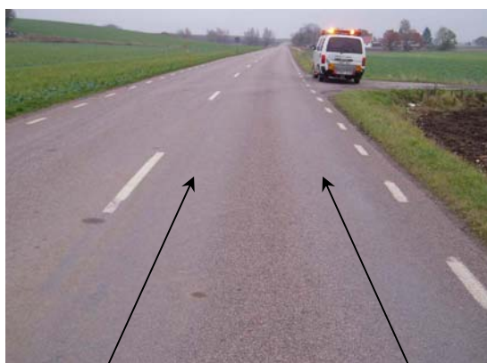
Fig 1: Part of road 1003 with obvious bleedings in the wheel paths
