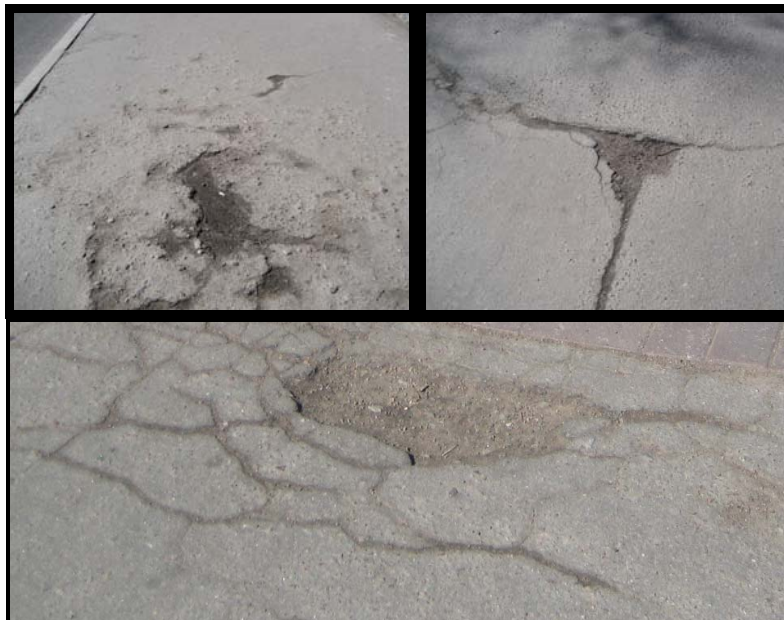
Figur 25. Cracks and holes on the pavement
