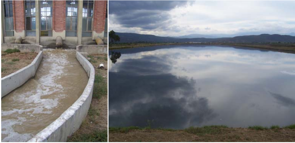
Figure 5. Wastewater pumping (left) and stabilization ponds (right) at Alba Rancho.
