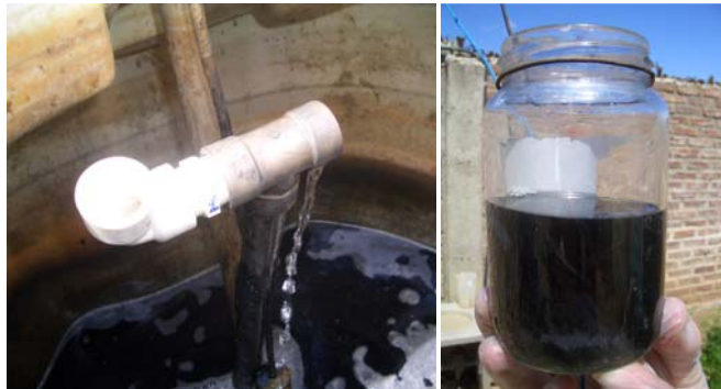
Figure 42. Left: effluent pipe. Right: water from effluent pipe.
