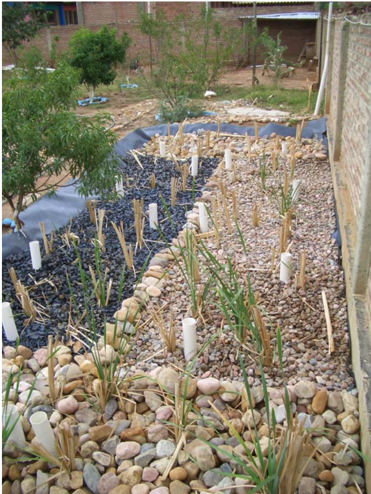
Figure 16. The HSF constructed wetland PTAR1. The black part is the plastic medium and the white tubes are observation pipes.
