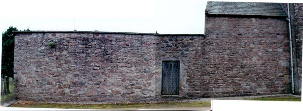
Figure 27: The north elevation of the extended chancel, now in use as the Lair of Grant burial enclosure. Photograph by Gertie Ericsson 1997.
