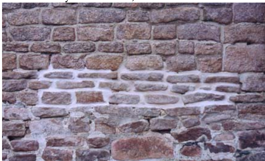
Figure 18: The south elevation of the tower, where repointing work was done in 1997. Photograph by Gertie Ericsson 1997.
