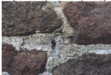
Figure 19: The south elevation of the tower where a piece of glass had been used as ballast in the masonry. Photograph by Gertie Ericsson 1997.
