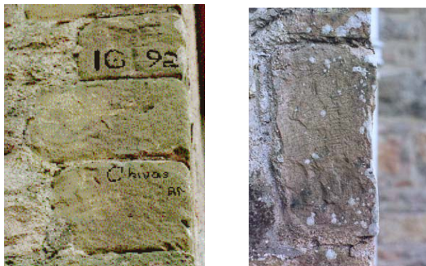
Figure 25: A few mason's marks on the northeast elevation of the nave, and chiselmarks on the northeastern quoin. Photograph by Gertie Ericsson 1997.
