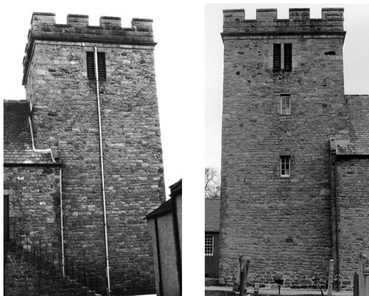
Figure 20: The north and south elevations of the tower. Photograph by Gertie Ericsson 1997.
