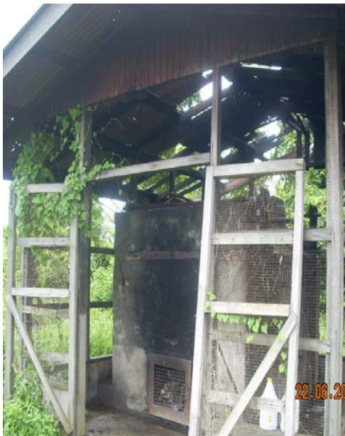
Existing furnace used for incineration of infectious waste at the West Demerara Regional Hospital
