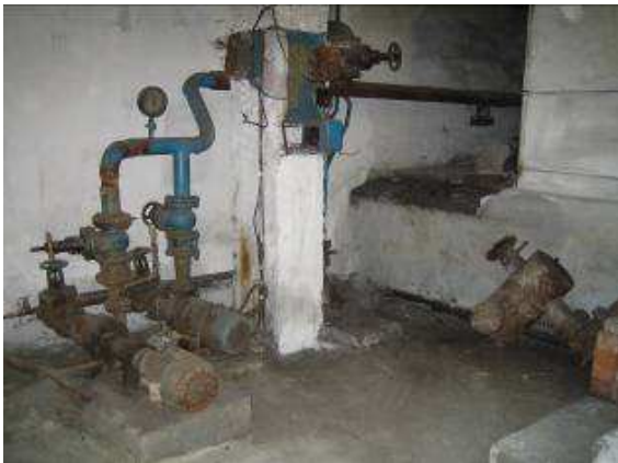
Figure 4-3 Nisporeni District Hospital. Old substation
