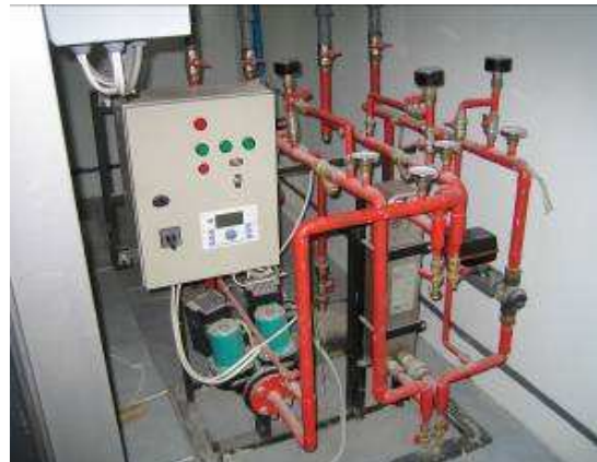
Figure 4-4 Nisporeni District Hospital. New substation
