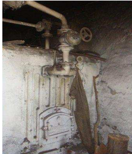
Figure 4-6 Soroca secondary school. Non-operating boiler
