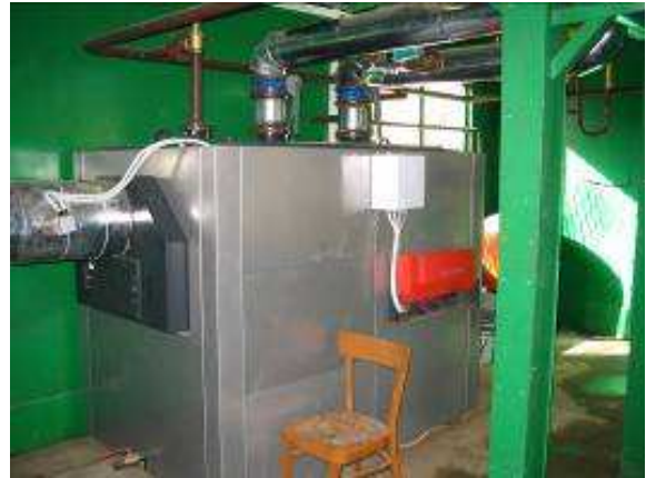
Figure 4-2 Leova District Hospital. New boiler
