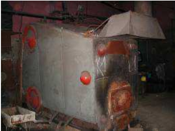
Figure 4-1 Leova District Hospital. Old boiler
