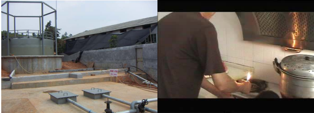
Figure 3-4 The biogas utilization facilities
