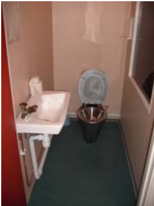
Another example of a toilet with washing facility at the police station in Sundsvall, Sweden. The window on the right side is for enable the custody officer to observe the detainee. The custody officer can see the detainee but the detainee cannot see the custody officer.
