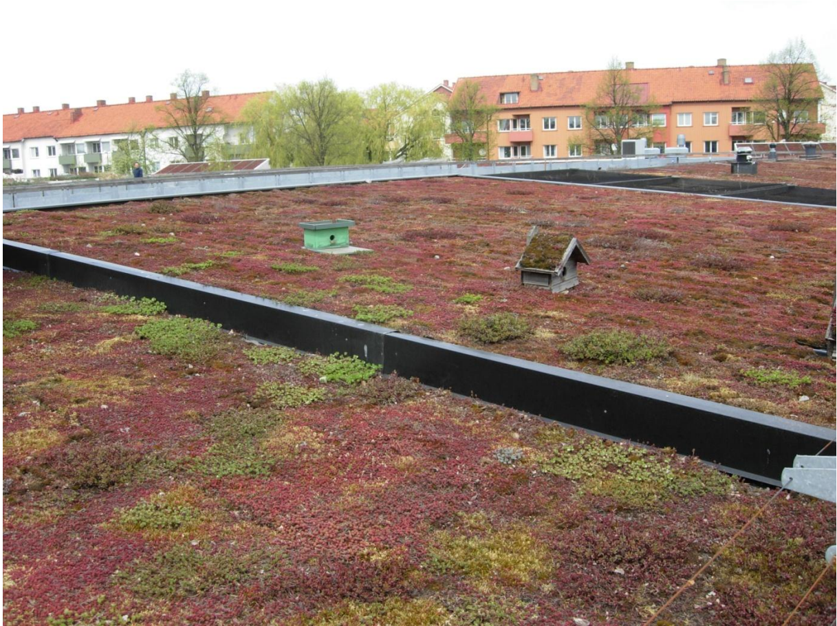
Picture (1). View on the green roofs in Augustenborg.
