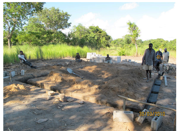
18- First day of the construction of the community house in Etaga (Pebane District)
