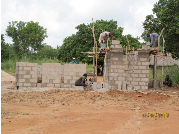
19- Second day of the construction of the community house in Etaga (Pebane District)
