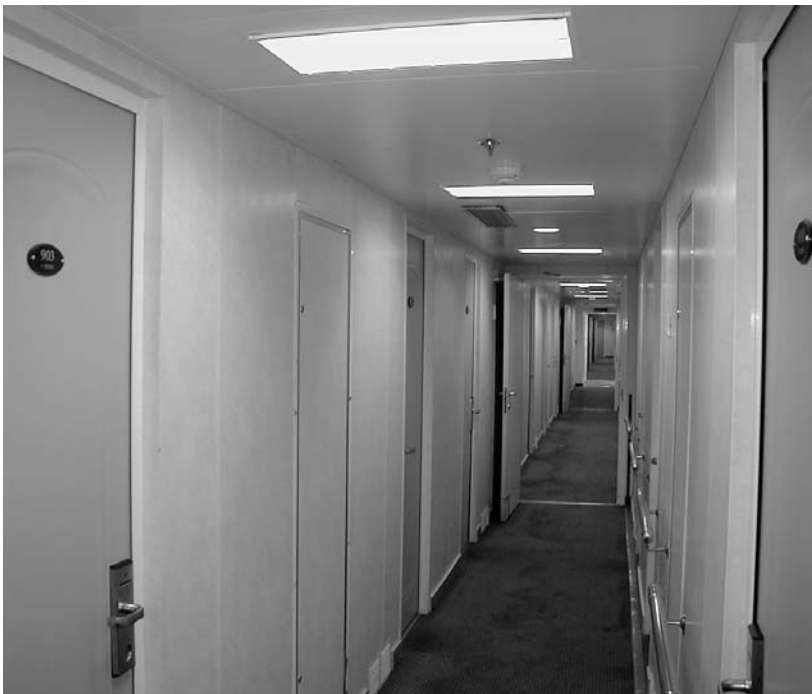
Figure 14: Doors dividing the corridor into three compartments.
