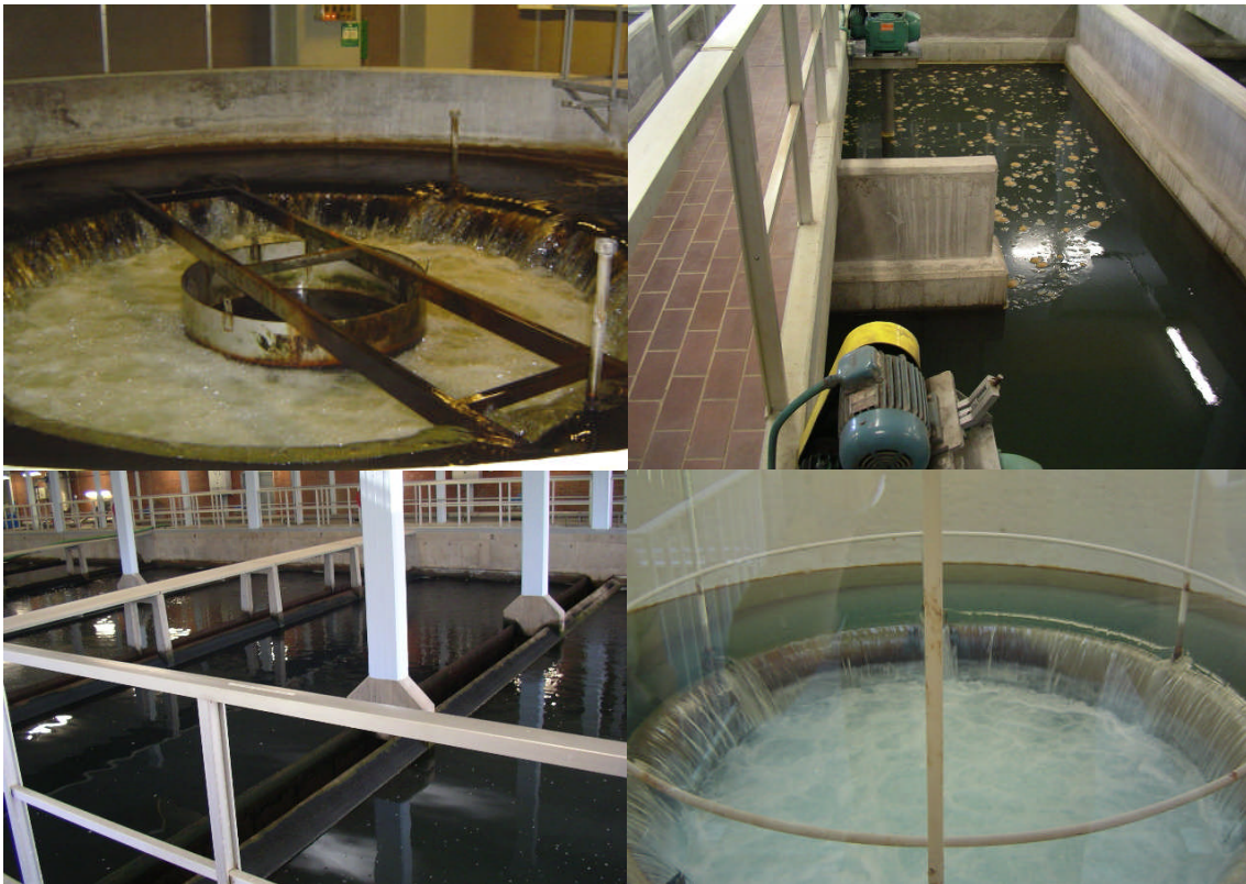
Figure 11. Upper left: raw water weir. Upper right: flocculation mixing chamber. Lower left: GAC filters. Lower right: drinking water weir.
