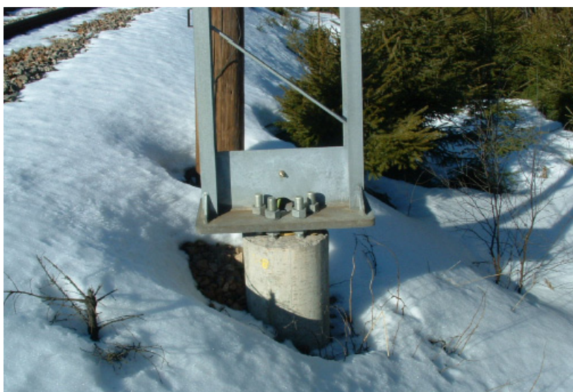
Figur 2.11 Kompletterat installerat MoFix-fundament (Stenman 2005, s.23)
