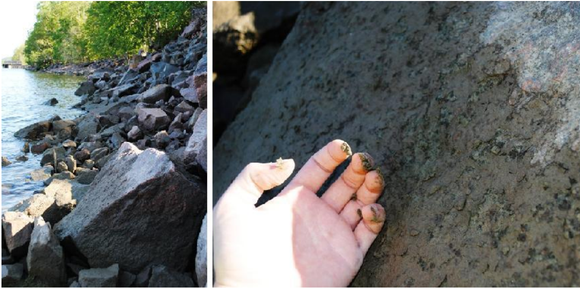
Figure 30 – Anthropogenic erosion protection at Garn station. The blocks and boulders are partly covered by fine cohesive sediment at times of low SWL, which is easily scraped off. This layer is thought to be easily eroded and consequently, to varying extent, also added as SPM to the river during times of precipitation. This could partly explain the prompt increase in mean turbidity in times of precipitation (© Althage 2010).
