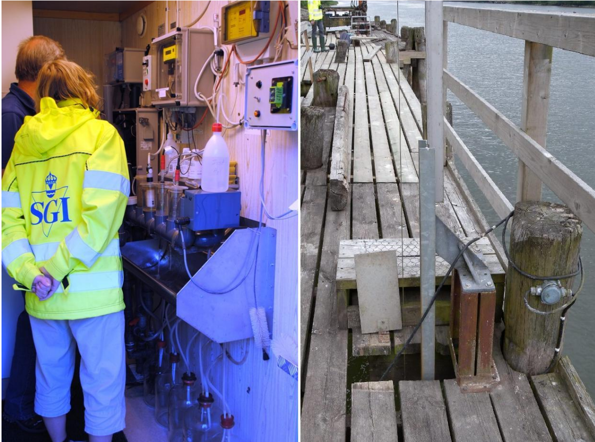
Figure 23 – Left; Equipment operated by Gothenburg water for continuously monitor the river water quality (© Althage 2010). Right; Location of the pump which supplies water to the monitoring equipment (© Göransson 2010).
