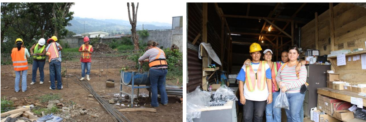
Figure 11. Everyone helps out with the construction. The women in the left image are working with the reinforcement and the women in the right image are working in the storage room. (2010-04-29)
