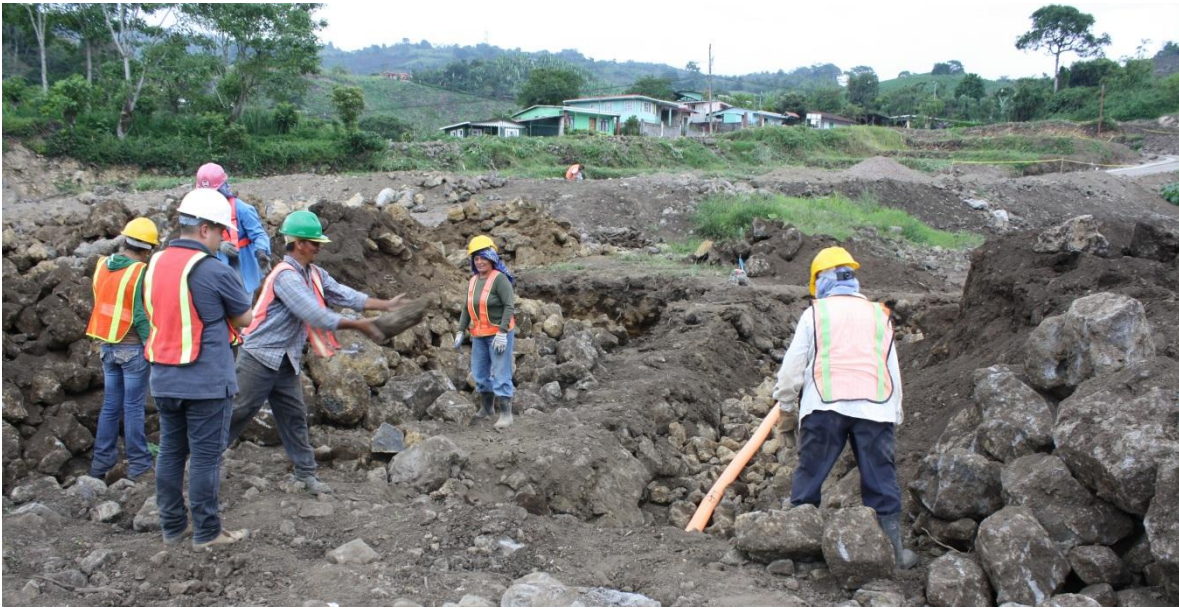
Figure 6. Preparatory work to lay the house foundation. The ground consists of dirt mixed with big rocks, which makes it solid but difficult to treat
