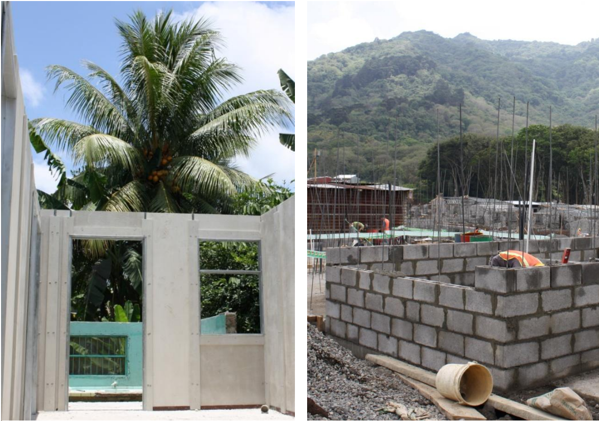
Figure 20. Left picture: framework made of fiber-cement boards in Puerto Limón. Right picture: framework made of concrete hollow blocks in the project Bethel.
