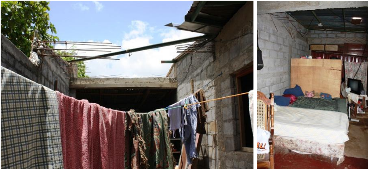
Figure 25. The family lives at the back of their shop. The reinforcement is sticking out from the joist prepared for the next addition that the family is planning to perform as soon as they receive the next loan from PRODEL.
