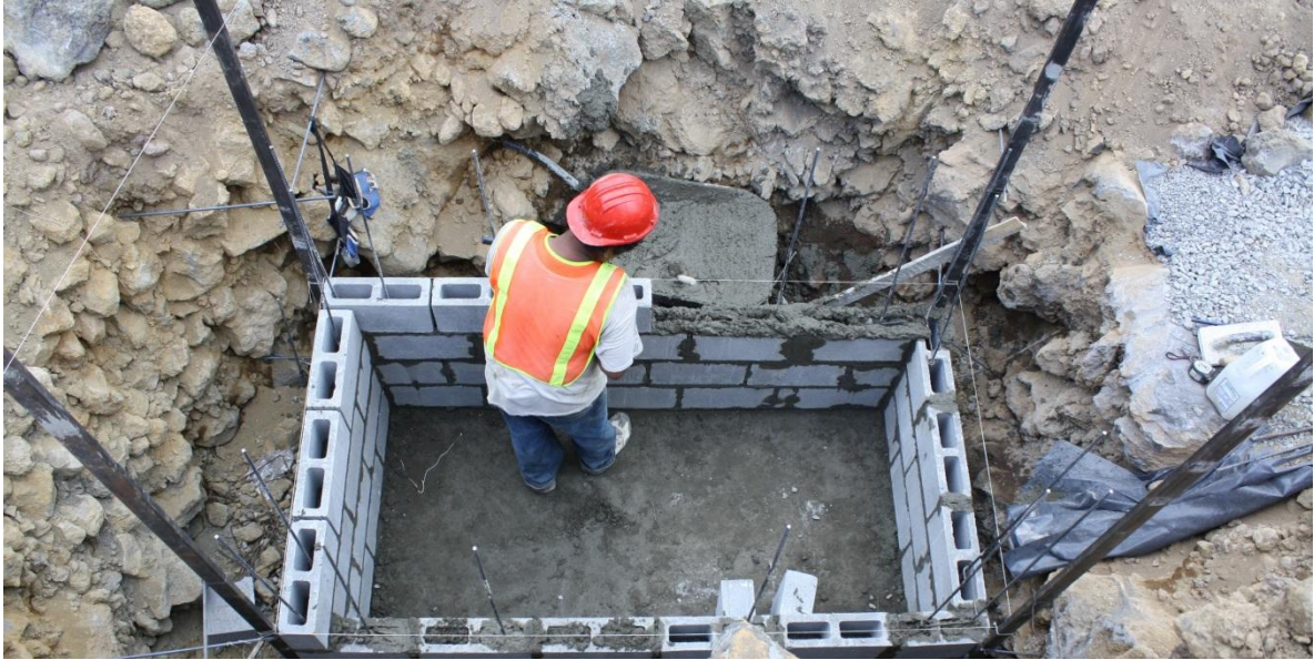
Figure 8. Preparation for plumbing and septic tank, people who work here will later move into the new houses that they have built themselves (2010-04-29)
