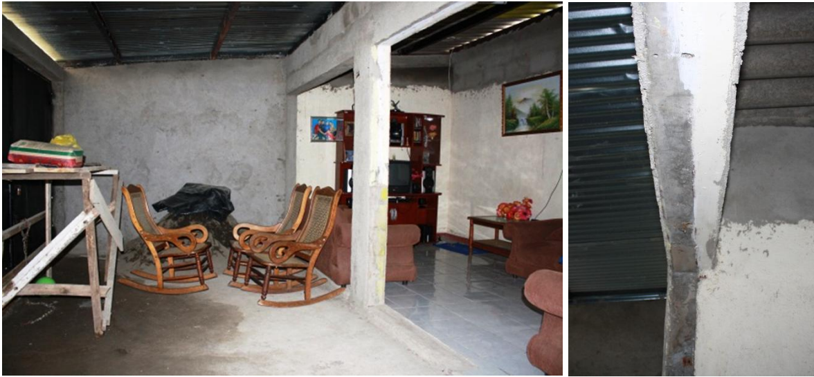
Figure 22. The left side of the room is the newly built extension. It is possible to see the old structure of the house by the white color on the wall in the right room. Previously there was no slope on the roof which prevented the rainwater from running off.
