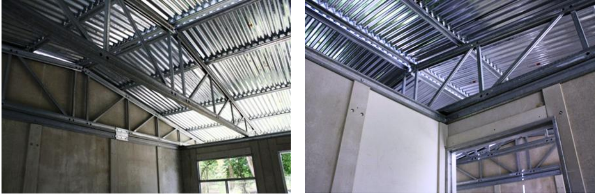
Figure 21. The roof of a house in Puerto Limón, with galvanized steel sheets mounted on the framework.
