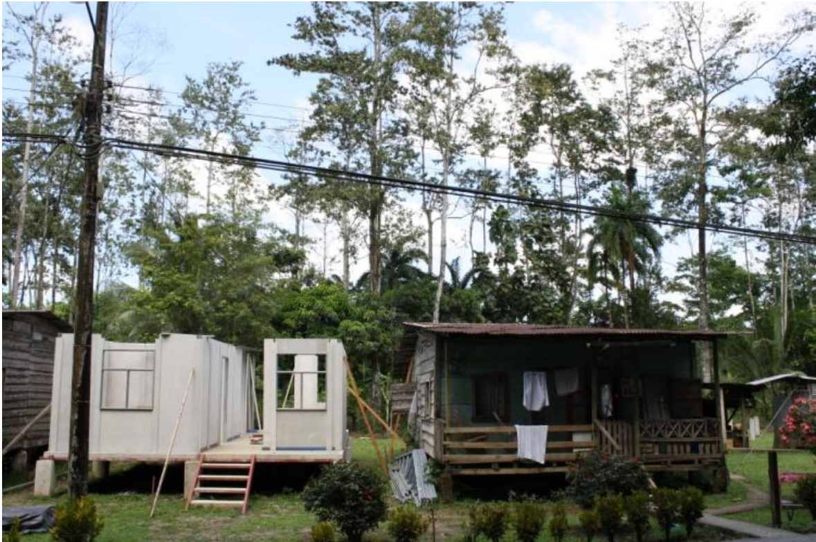
Figure 17. The project consists of six individual houses that are first demolished, then rebuilt. Above is an illustration of the possible changes.
