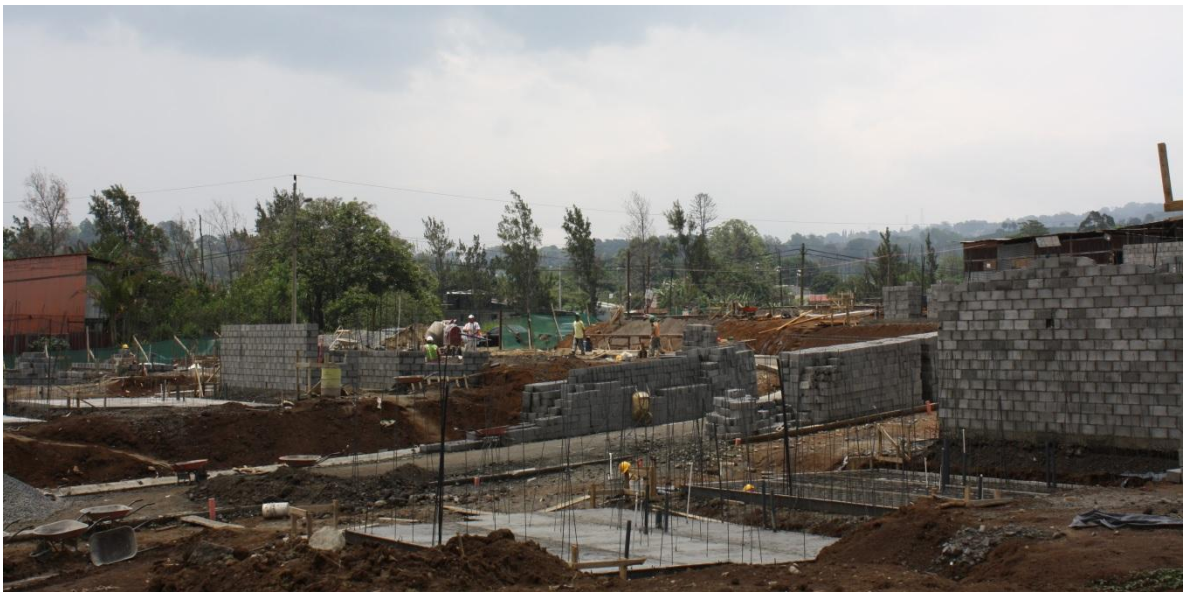
Figure 9. The building site is divided into nine separate zones. The division makes the construction more efficient and facilitates its management.
