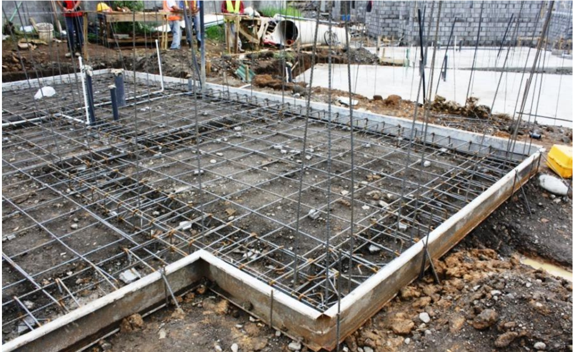
Figure 19. A commonly applied technique for the foundation is ground slab. Large amounts of reinforcements are installed to prevent possible collapse. (2010-04-29)
