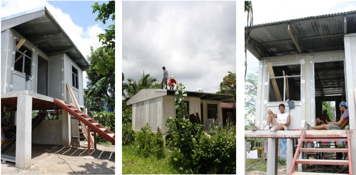
Figure 18. The houses are built on concrete pillars to protect the house from regular flooding. The height of the pillars depends on the amount of water that strikes the area. (2010-04-23)
