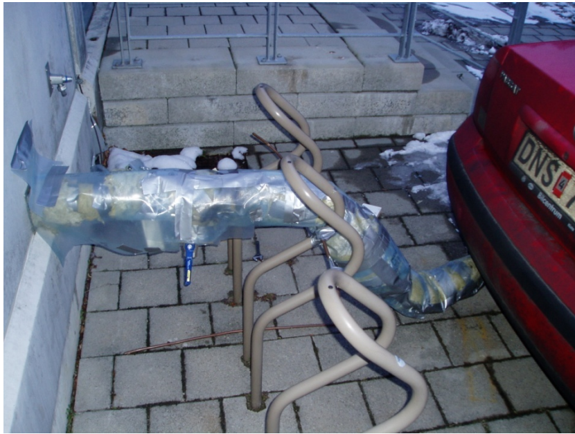
Figure 5.2. The exhaust extraction system.
