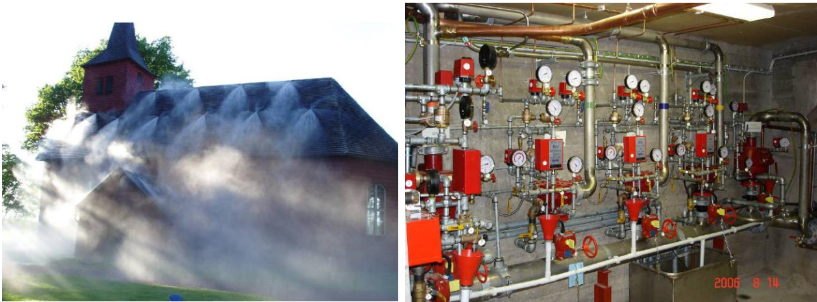
Figure 2.5 Left: functional test of a deluge water mist sprinkler system for external roof and facade protection of Älgårås church in Sweden. Right: deluge and dry pipe valve assembly for similar system in Habo church, Sweden. (Arvidson, 2006)
