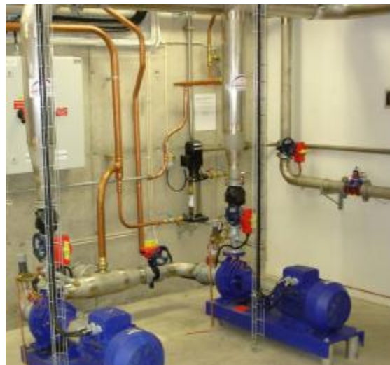
Figure 3.10 Electrical centrifugal pumps supplying a conventional sprinkler system with water, (Arvidson, 2006)
