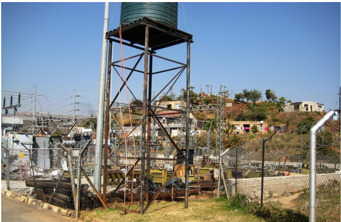
Figure D.4 - Settlements in the vicinity of the electrical power plant, Kabokweni.
