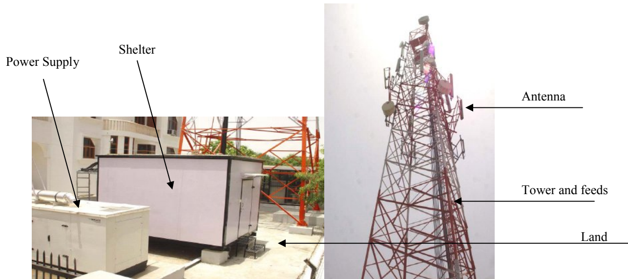
Figure 4.2. One of the first Indian sites which have implemented the shared infrastructure concept.
