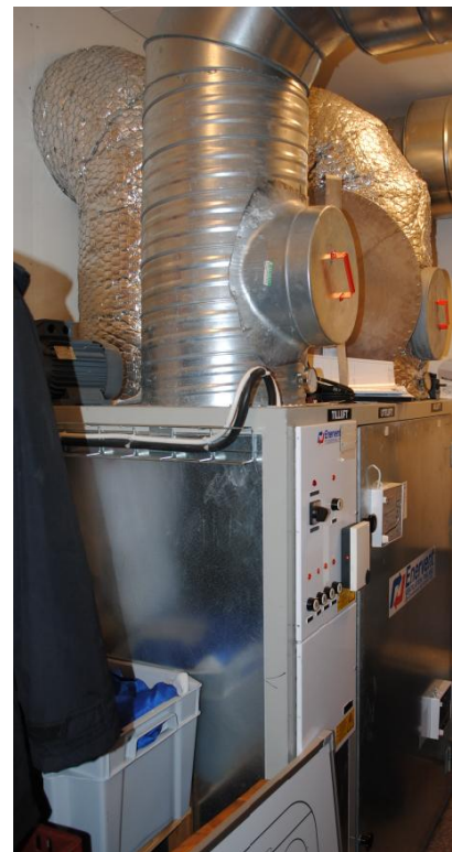
Figur 2.14 – Ventilationsaggregatet i brandcell 2.
