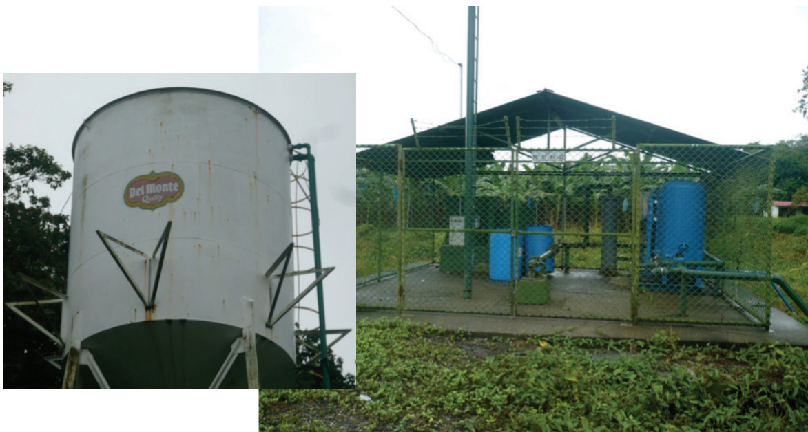
Figure 7. Water tank and well for drinking-water extraction in Bananita.
