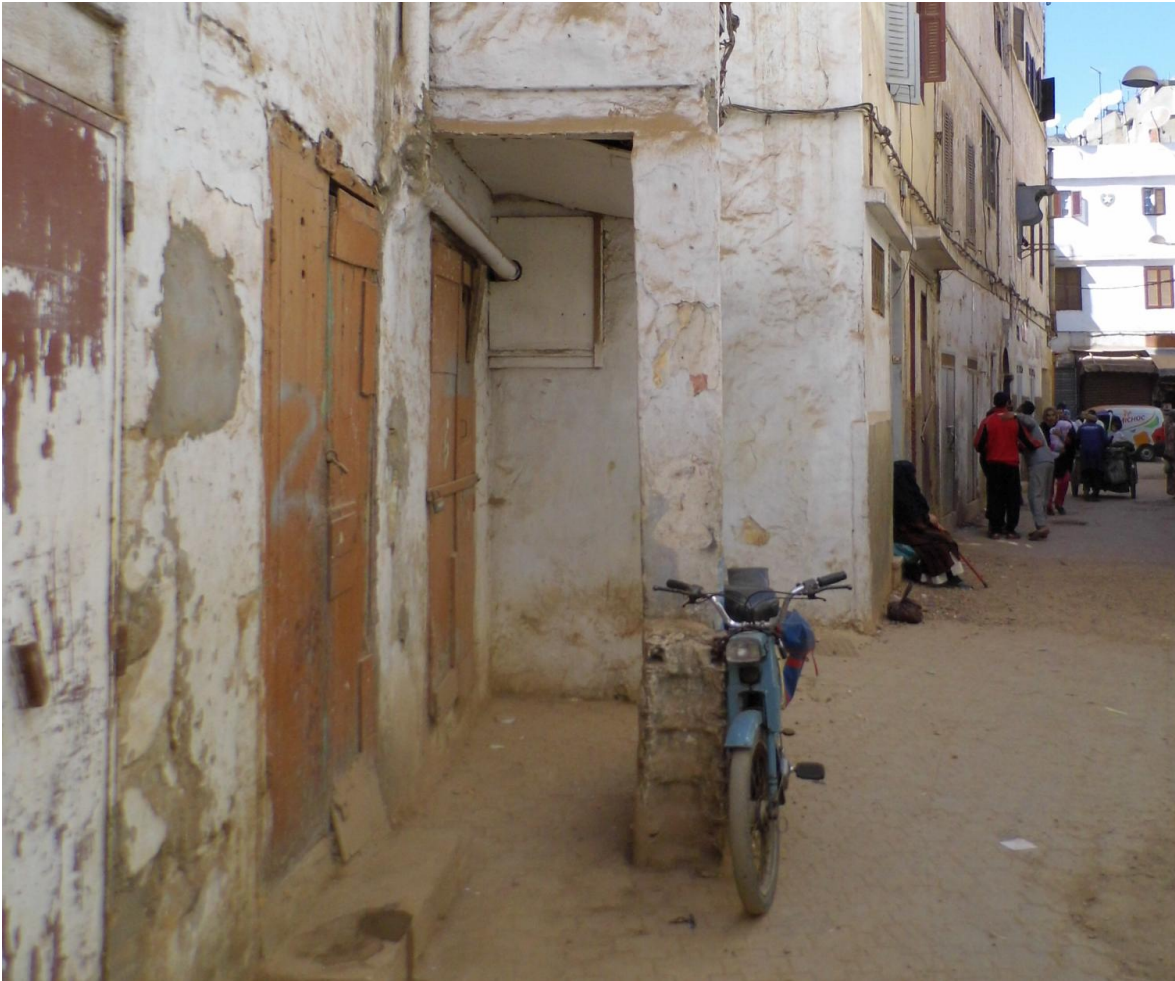
Fig 13. A crocked pillar, holding up an extension of the first floor.
