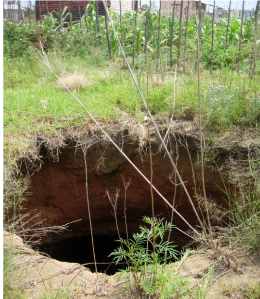
Figure 15. Sink-hole with a shack in the background.
