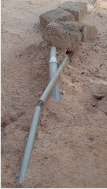
Figure 3. PVC-pipes above ground surface in Yaase. Photo: Kristoffer Ristinmaa
