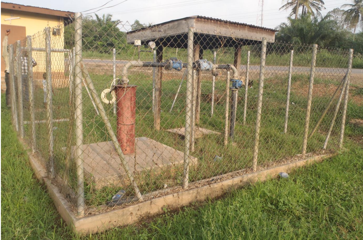
Figure 2. A mechanized borehole in Kuntanase with fence to prevent intrusion by animals. The yellow building in the background is the related pump house. Photo: Kristoffer Ristinmaa
