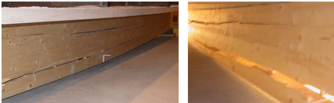
Figure 3.3: Failure of one of the timber beams.
