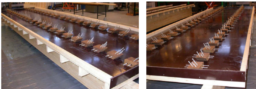
Figure 3.1: Formwork before the casting of the concrete with the connection system F45.
