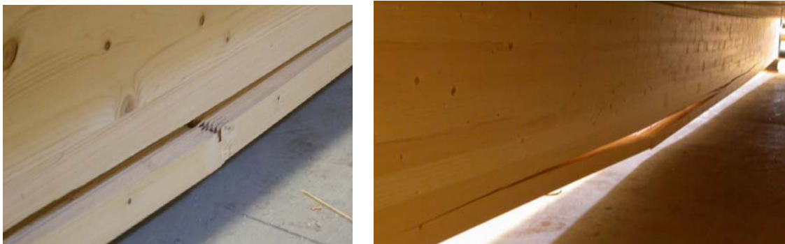
Figure 3.11: First failure of the office floor due to the breaking of one finger joint in one timber beam.
