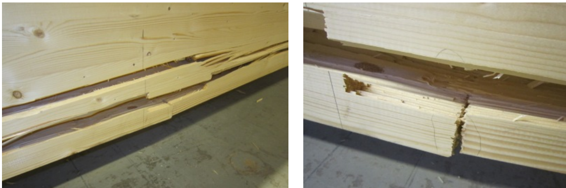
Figure 7.20: Failure of the floor system due to the breaking of one finger joint in one timber beam.
