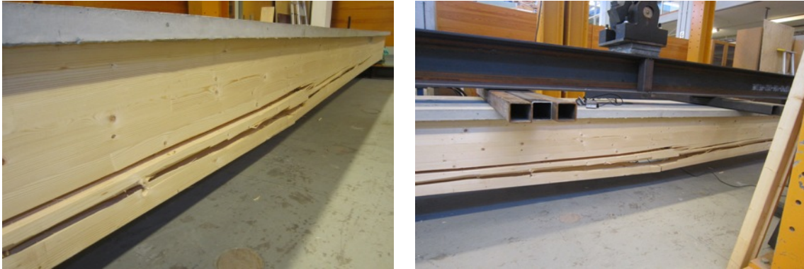
Figure 7.19: Cracks along the failure beam A2.
